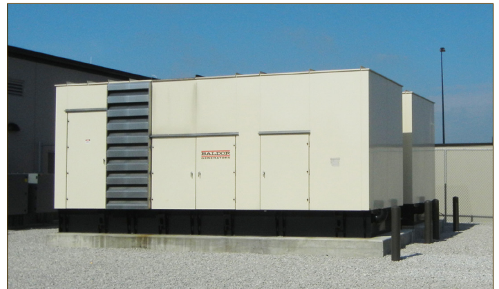
Figure 7. Two 1-MW generators provide emergency power to the data center in the event of a utility outage. The units can be operated separately or in parallel, as needed. A PLC controls the generators, utility power, UPS units and a battery farm.
