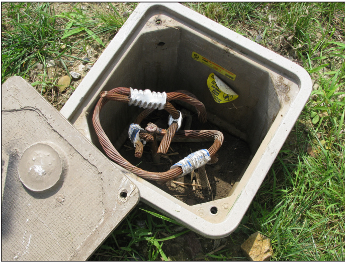
Figure 13. A 500-MCM bare copper ring-ground runs along the periphery of the data center structure. Grounding conductors from the MGB, the rooftop lightning protection system, the substation yard and the transformer yard are bonded to the ring, which serves as the single common reference grounding point for the entire data center.
