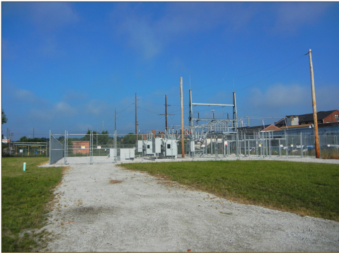
Figure 5. With only one utility serving its Akron location, Involta elected to build its own substation adjacent to its data center. Redundancy is achieved by having duplicate breakers, transformers and switchgear for A and B circuits.
