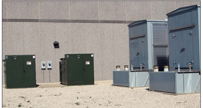
Figure 2. Involta-Marion's two independently fed 2500-kVA utility transformers are seen at left. Two of the center's four 750-kVA diesel generators are visible at right. Either of the transformers and any three of the generators can fully power the data center. Additional generators can be added as the data center expands. Not visible in the photo is a buried web of 4/0 AWG copper grounding conductors that connect all equipment and the switchyard's fence into the center's single-point grounding system.
