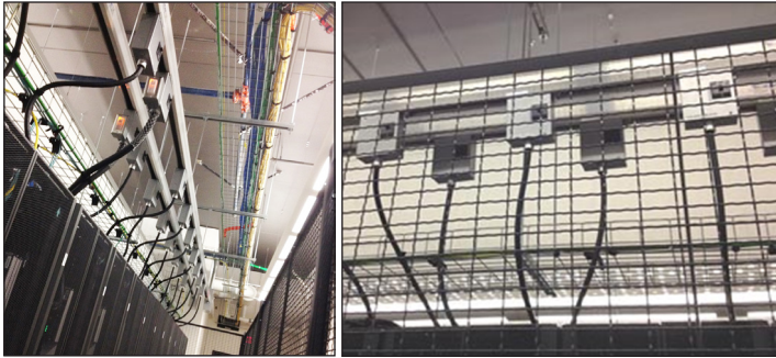
Figure 8. Power is fed to racks via overhead Starline busways (left). Both A and B circuits run in the busways, but the photo at right shows their separate feeds to the racks.
