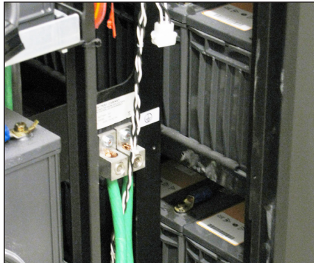
Figure 9. Dual grounding conductors are shown bonded to a rack in one of the center's battery farms. The green wires are routed upward to a cable tray, and from there to a ground bar mounted on a nearby wall.
