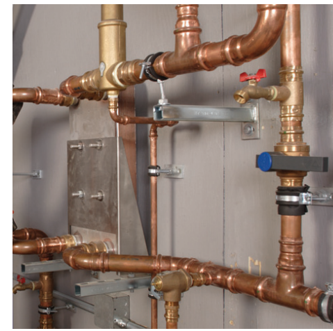
Copper system installation, courtesy of Viega, LLC
