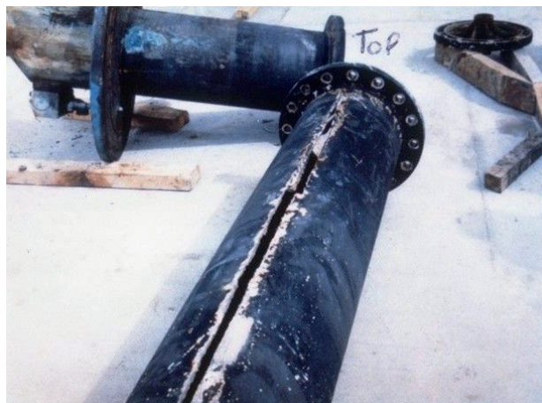
Figure 10 - Corrosion of nickel aluminium bronze pipe along seam weld due to residual beta-phase
